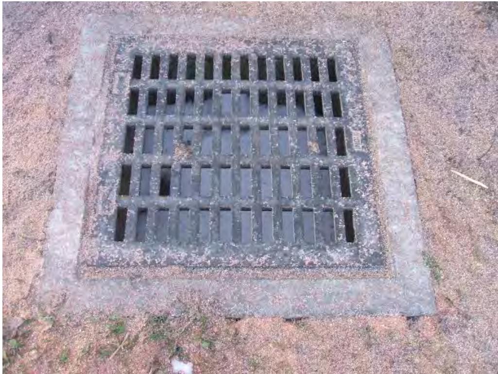
Photo #21: View of an exterior storm water drain.
